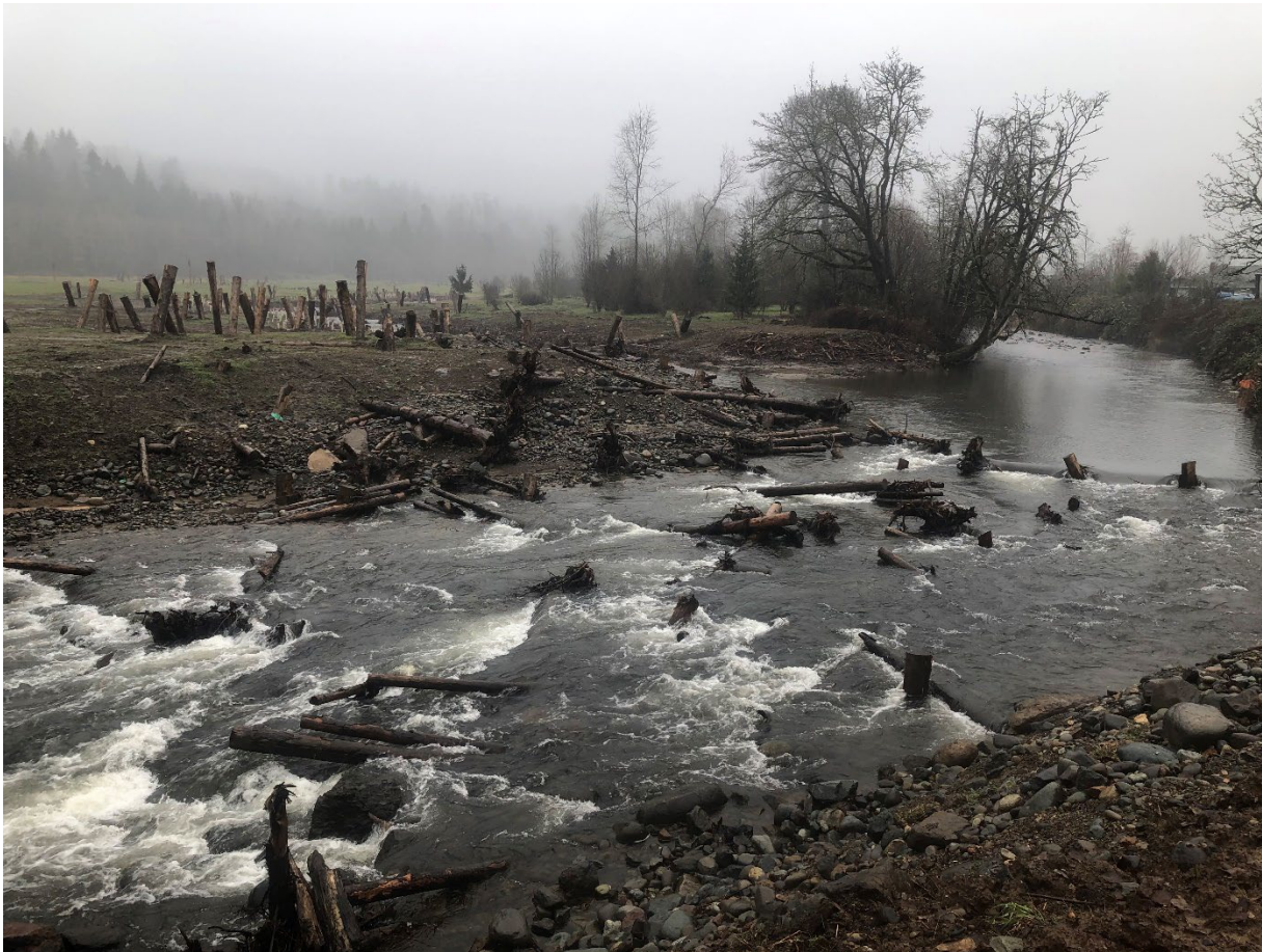
Figure 10-6 Example of Large-Channel Wood Grade Control
