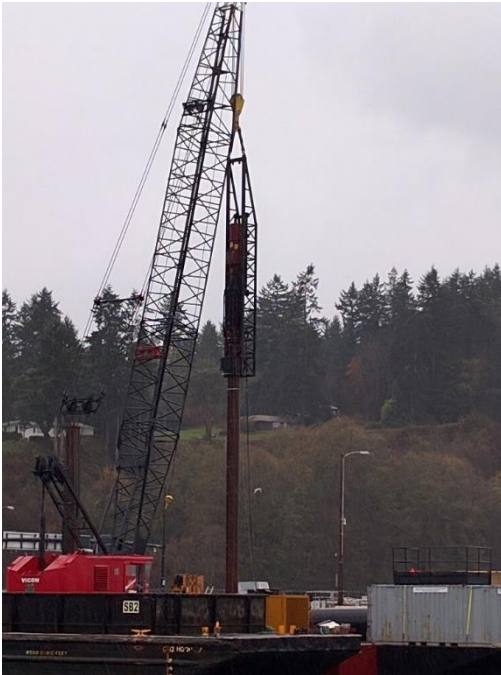
Figure 3a. Photograph of the placement of the impact hammer on the control pile taken from the R/V Robertson on 7 December.
