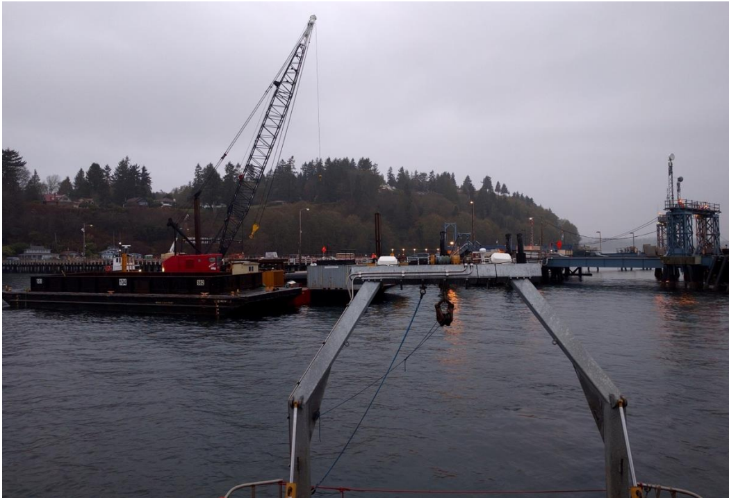
Figure 2a. Photograph from the stern of the anchored R/V Robertson overlooking the A-frame and looking towards the construction barge complex, taken at 9:00 am on 7 December.
