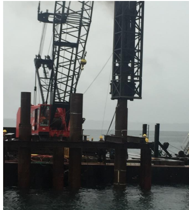
Figure 3b. Photograph of the three piles in the template taken on 8 December. The control pile is on the left, the double wall pile is in the middle, and the mandrel pile is on the right.
