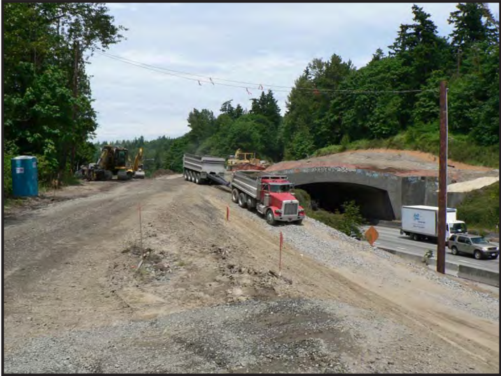
Figure 60. Wilburton Tunnel in 2008 prior to demolition, view to the north. Note southbound I-405 traffic beneath the overpass. (Photograph courtesy of Tom Doolittle, Doolittle Construction.)
