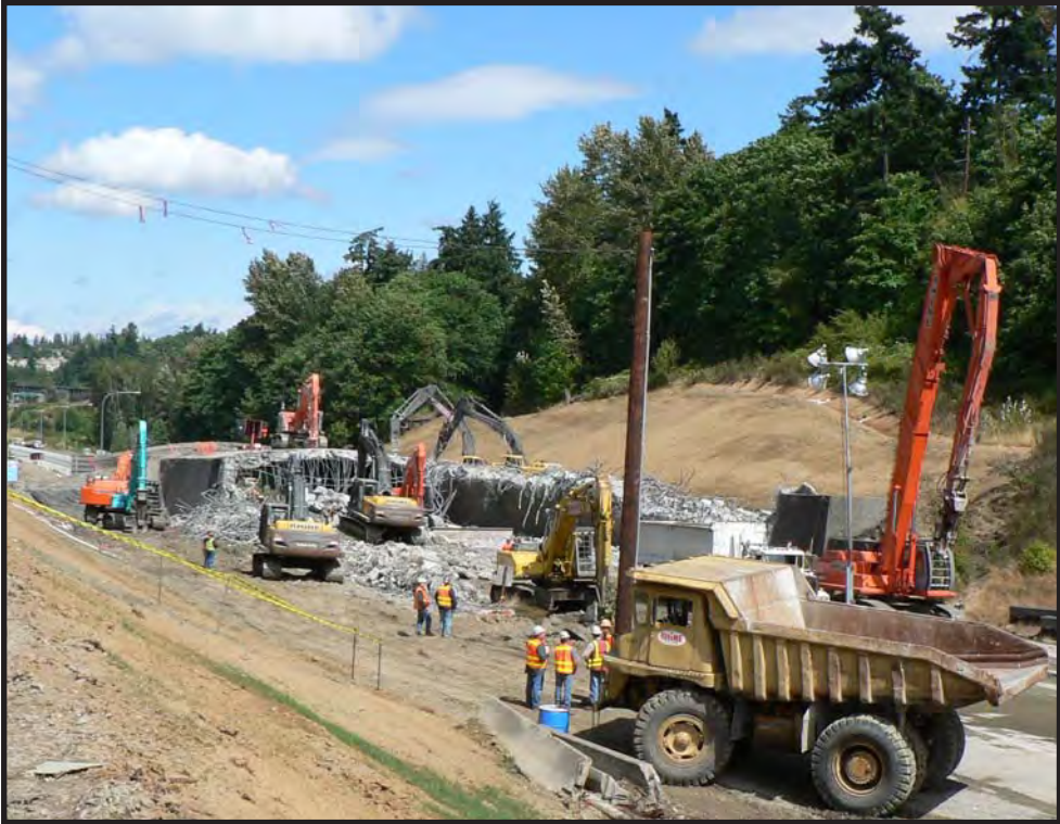
Figure 61. Wilburton Tunnel demolition in 2008, the view is to the north. (Photograph courtesy of Tom Doolittle, Doolittle Construction.)
