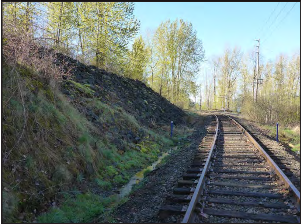
Figure 44. Northern Pacific Lake Washington Belt Line, riprap slope along railroad tracks in Zone 49, view to the southwest.
