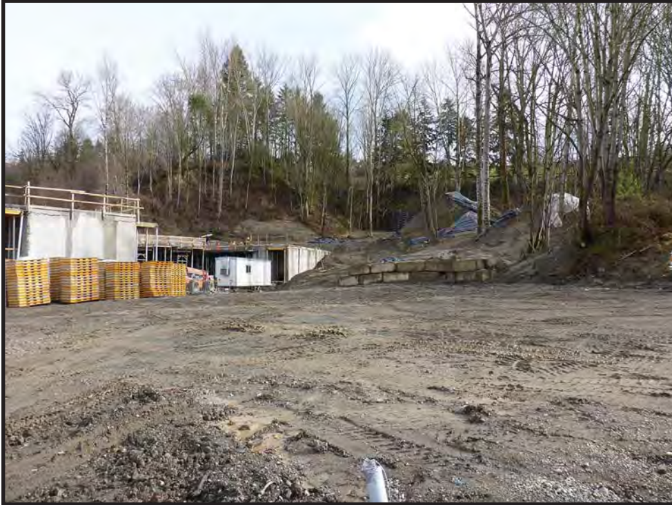
Figure 4. The area adjacent to Zone 18, showing ongoing commercial or residential construction to the east of Lake Washington Boulevard near the entrance to Gene Coulon Memorial Park. View to the east.
