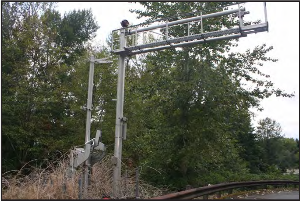
Figure 53. Grade crossing at Lake Washington Boulevard, signal gate, view to the northeast.
