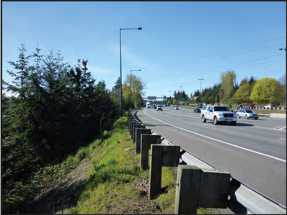
Figure 32. Elevated fill slope on the eastern edge of I-405 typical of Zone 61. View to the southwest.
