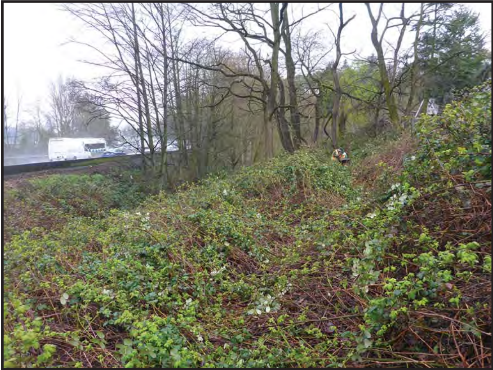
Figure 21. The densely vegetated slope in Zone 42 is shown in this photograph to the north.
