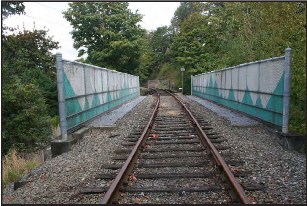
Figure 49. Future Lake Washington Boulevard bicycle trail bridge, deck, view to the north.
