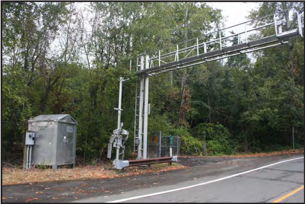
Figure 54. Grade crossing at Lake Washington Boulevard, signal gate and utility building, view to the north.
