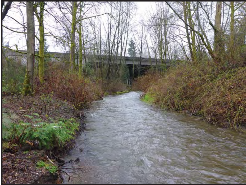
Figure 10. Zone 30, which includes May Creek to the west of I-405, is shown in this photograph to the southeast.
