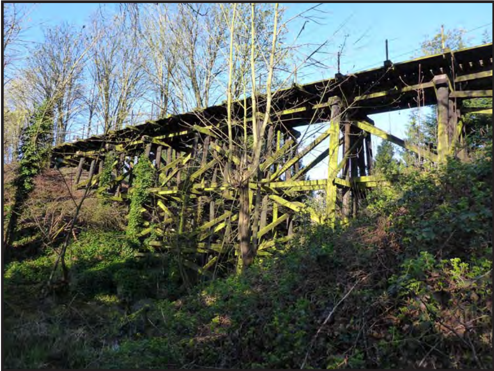
Figure 43. Northern Pacific Lake Washington Belt Line, trestle over Coal Creek in Zone 58, view to the southwest.
