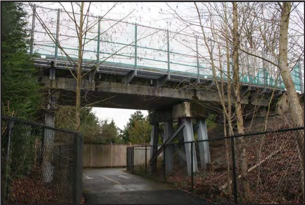
Figure 48. Future Lake Washington Boulevard bicycle trail bridge, underpass, view to the northwest.
