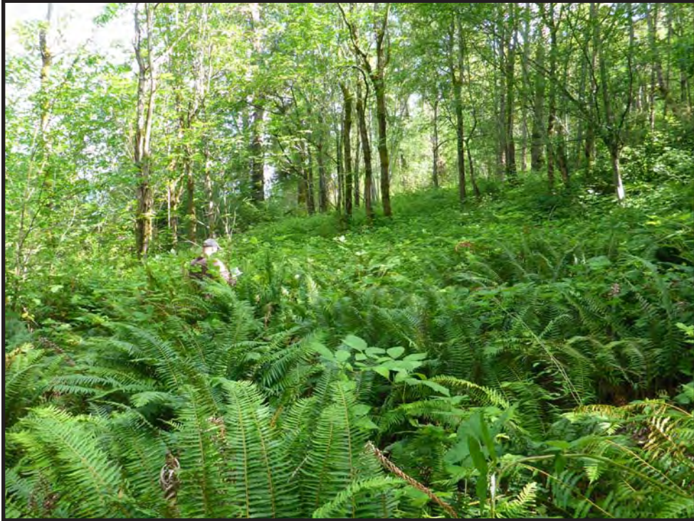
Figure 28. Zone 52, a broad, sloping terrace above the cut for the northbound lanes of I-405. The crew is excavating ST 205 in this view to the north.
