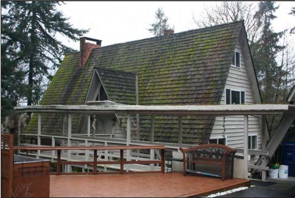
Figure 41. Paukstis house, 11620 SE 45th Place, south (front) and east elevations. The view is to the northwest.
