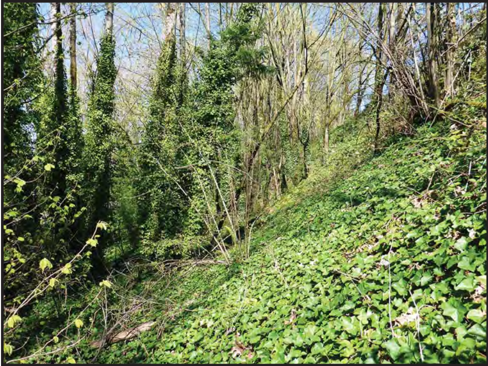
Figure 13. The steeply sloping road fill prism below (west of) I-405 southbound lanes in Zone 35 is shown in this photograph to the north.
