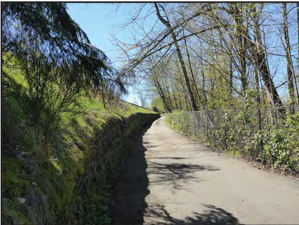
Figure 27. A paved bike path in northern Zone 49 (from the entrance of Newcastle Beach Park north to Coal Creek Parkway) is shown in this photograph to the south. Rock gabions support the fill slope below I-405.
