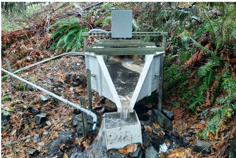
Figure 5 Mirrormont Influent Monitoring Equipment
